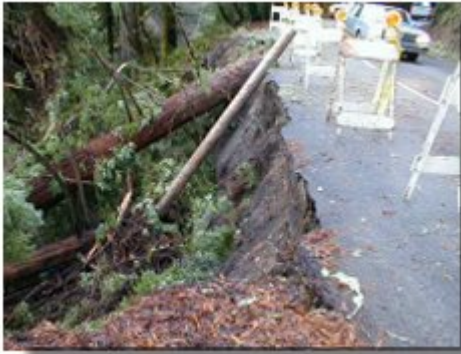
Mudslide Damaged Pope Road
