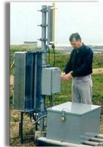
Equipment will be Vaulted with San Mateo Sheriff's Equipment
